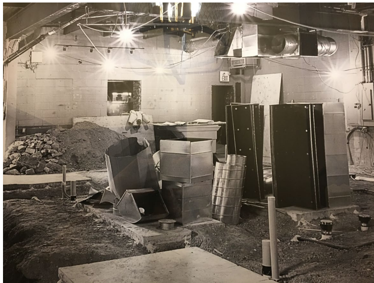
Photography in the washrooms provide a rough idea of just how much work was involved in getting The Burren ready. Pictured above is the effort to re-concrete the floors from mid-January, 2019
